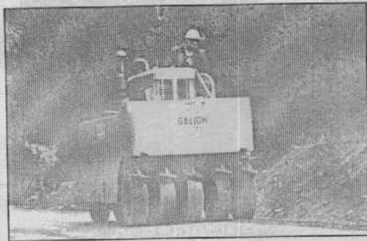
Pneumatic roller being used to compact sand base for a highway. (Courtesy of Galion Division of Dresser Industries, Inc.)
