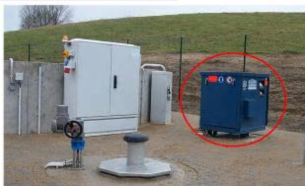
Blower for fine bubble aeration
